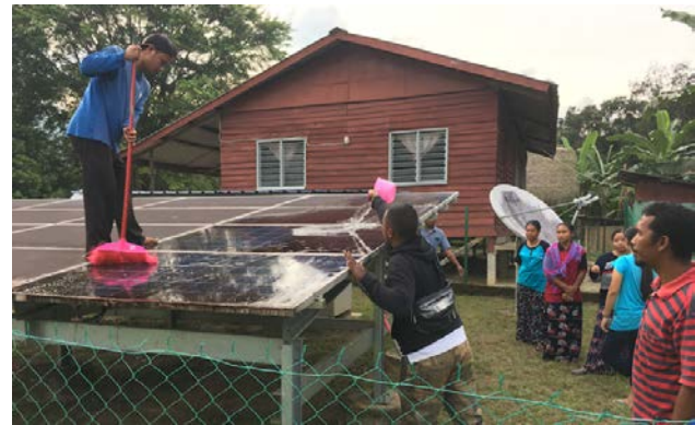
Fig. 4. Routine Communal Work of Cleaning the Solar Panels.
