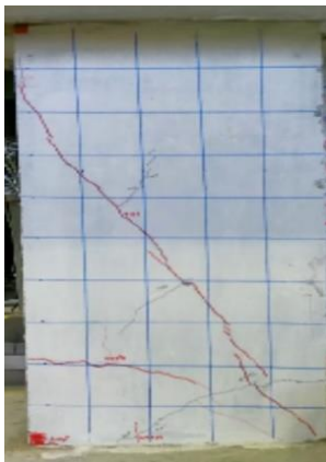
Fig. 3. Input image for crack detection.
