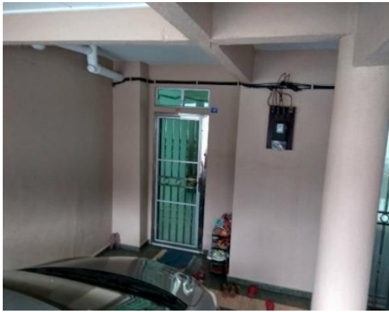
Fig. 13. Security Camera Facing Main Door.
