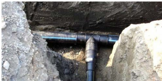
Fig. 3. Example of How a Private Branch is Actually Connected to the Distribution Pipe.
