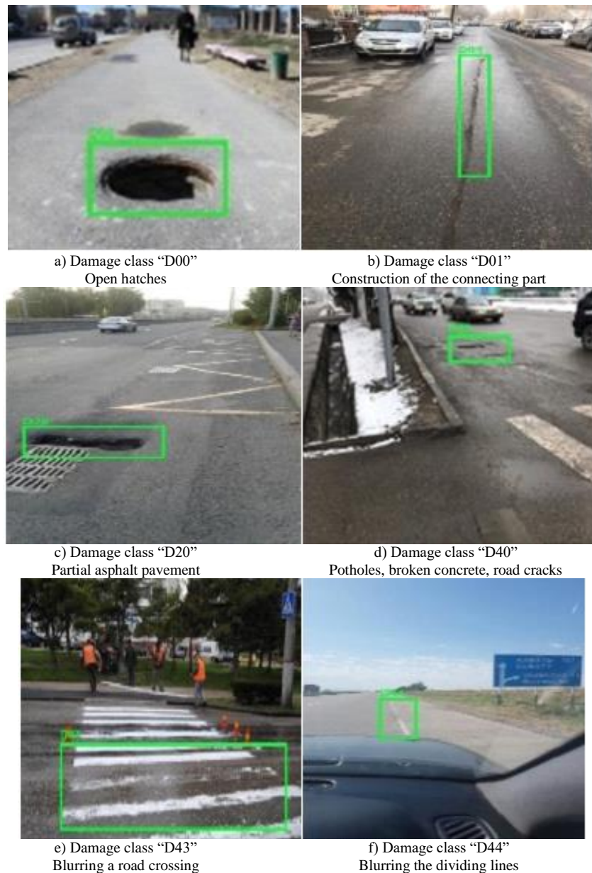
Fig. 1. Road damage photos and classes for a model training.
